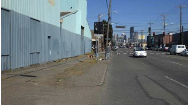
Example of poor condition of sidewalk and driveways, including driveways no longer in use.
